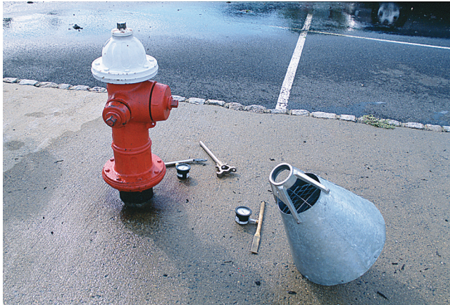
EXHIBIT 22 Diffuser — Slot for Pitot Tube Insertion.
