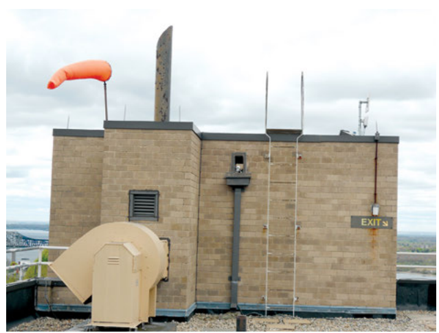
Fire escape ladder for rooftop access and egress.
