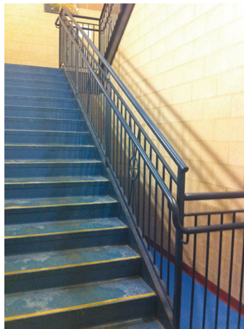
Permanent barricade installed to prevent storage beneath stair run.
