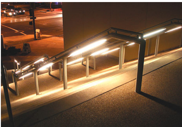
Exterior stair illumination via lights in stair handrail. (Photo courtesy of Jake Pauls)
