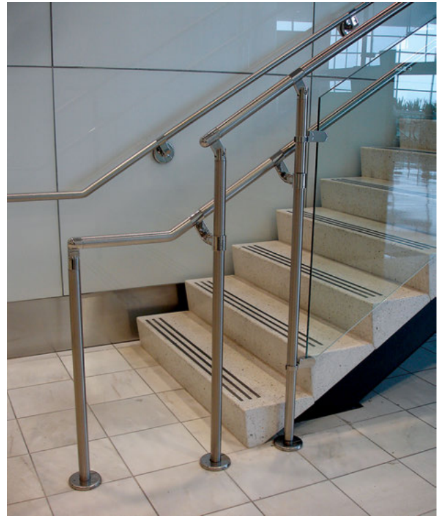
Stair with handrail extension at bottom of flight to alleviate user bunching. (Photo courtesy of Jake Pauls)
