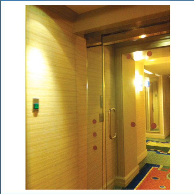
Circular decals that call attention to glass door in corridor egress path.
