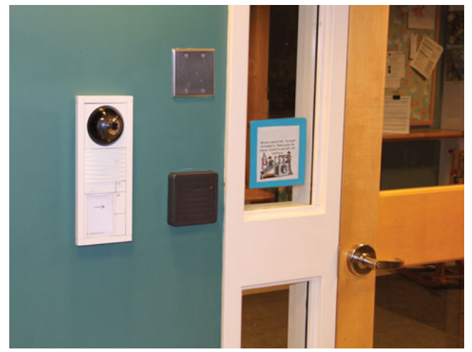
Security equipment associated with restricted entrance to day-care occupancy.
