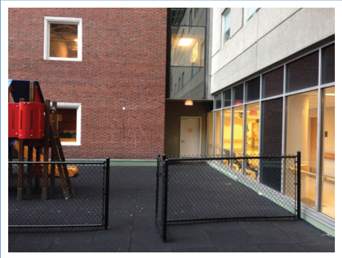
Door with delayed-egress hardware in second means of egress route.
