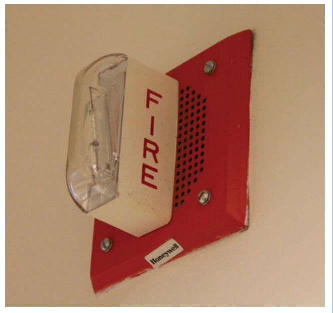
Horn and strobe for occupant notification.
