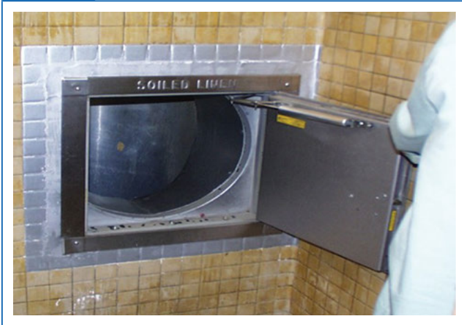
Linen chute opening.
