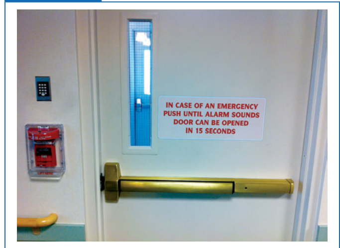
Delayed-egress locking hardware on door connecting corridor to exit enclosure.
