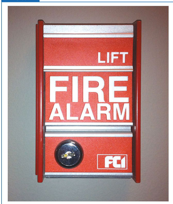
Typical manual fire alarm box.
