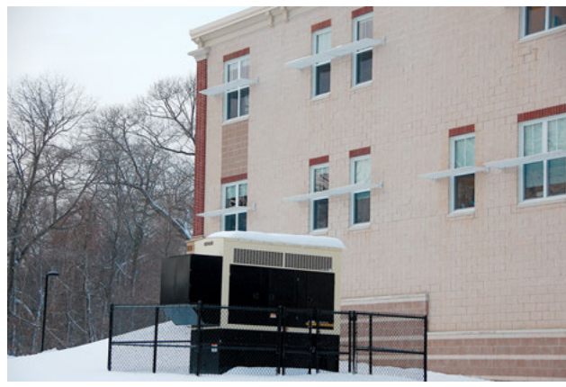
Emergency generator for emergency lighting.
