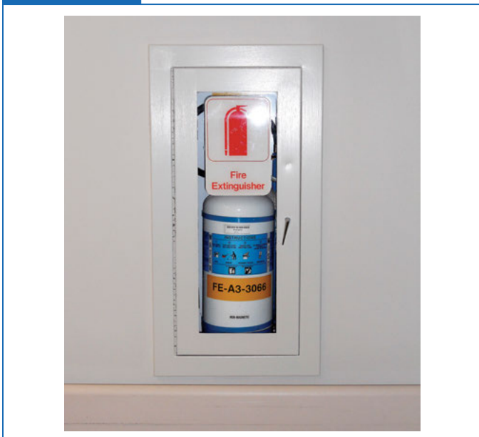
Portable fire extinguisher located in corridor of patient treatment area.
