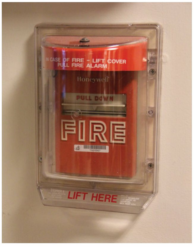
Manual fire alarm box with protective cover.
