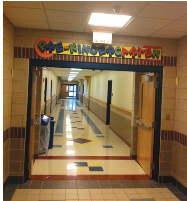
Cross-corridor doors in smoke barrier.
