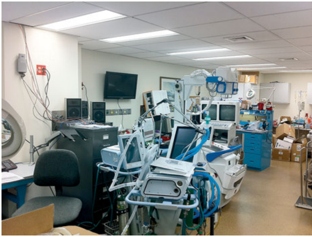
Medical equipment servicing room.
