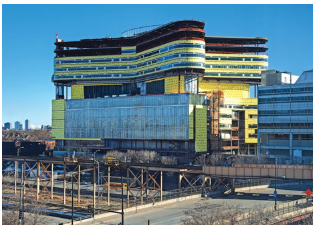
New construction (East Tower of Rush University Medical Center in Chicago, IL). (Courtesy of Leo T. Garcia, Rush Photo Group)
