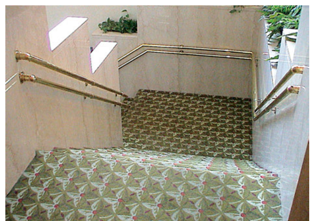
Additional handrail mounted at lower height than standard handrail. (Photo courtesy of Jake Pauls)
