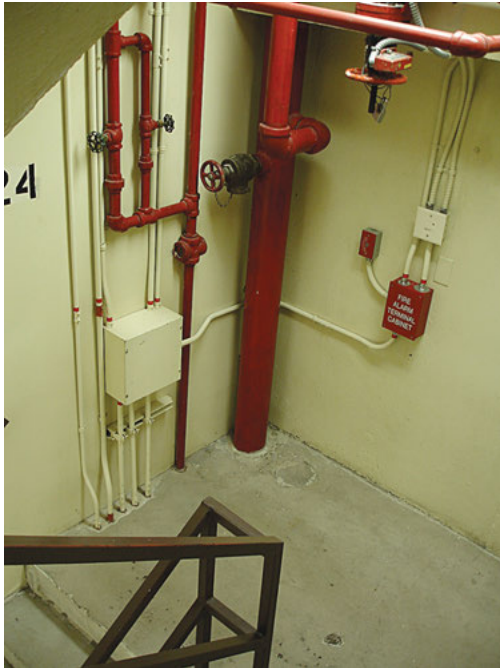
Fire protection and alarm equipment within, and penetrating the barrier walls of, an exit enclosure. (Photo courtesy of Jake Pauls)
