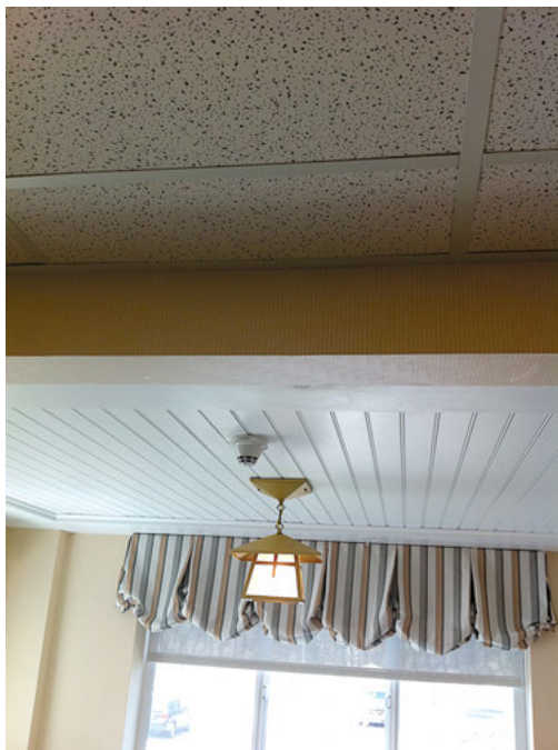
Smoke detection for space open to corridor but not readily supervised by staff.
