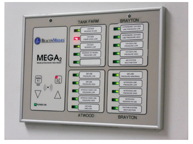
Medical gas monitoring panel.
