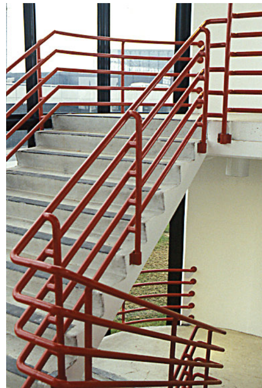
Horizontal rails in guard system that facilitate climbing. (Photo courtesy of Jake Pauls)
