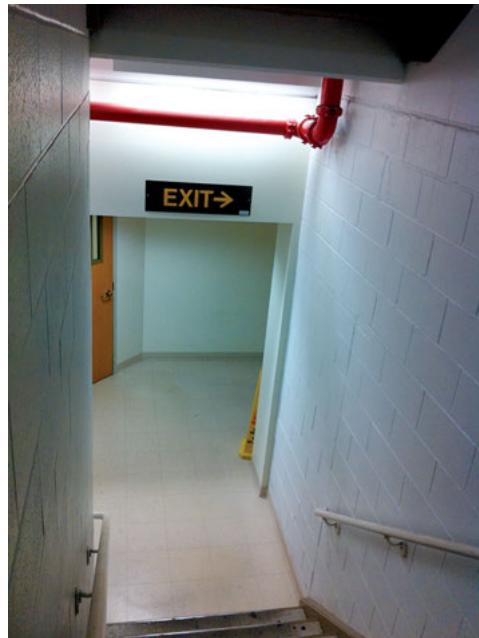
Directional marking within a horizontal component of the egress path within an exit enclosure.
