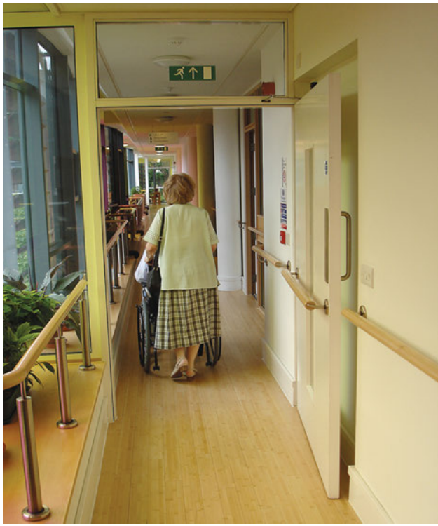
Permitted handrail encroachment on required corridor width. (Photo courtesy of Jake Pauls)
