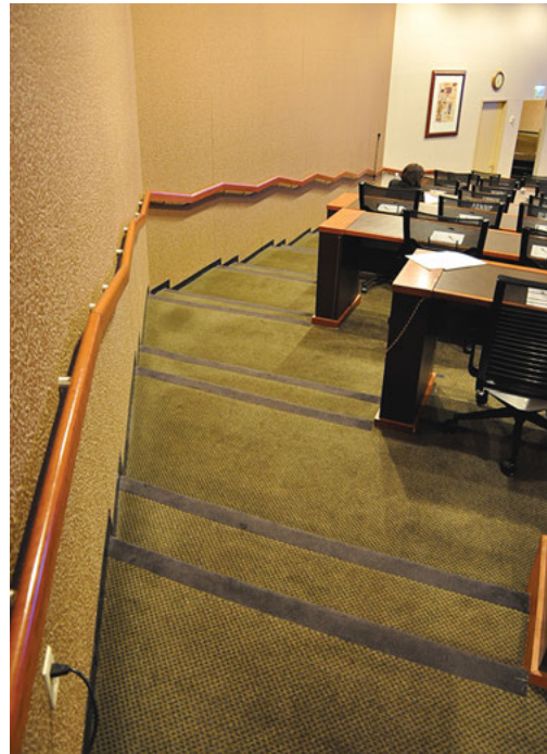
Stepped aisle nosing marking using permanent flooring material. (Photo courtesy of Jake Pauls)
