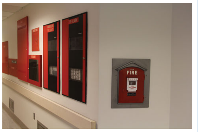
Auxiliary fire alarm box for emergency forces notification.
