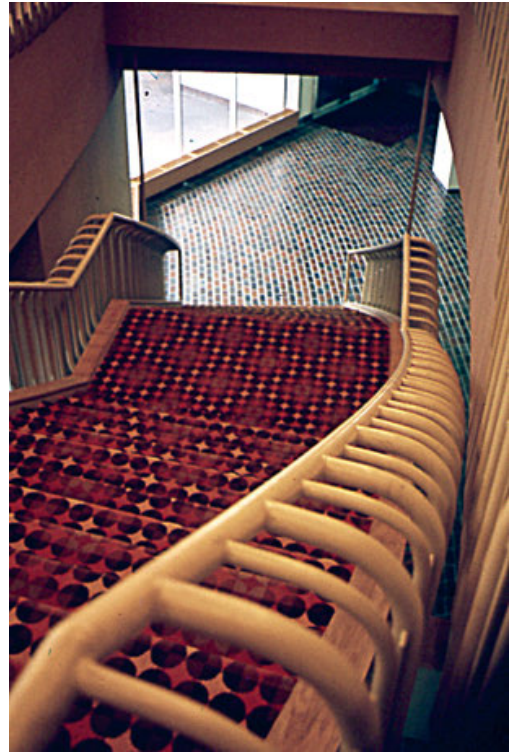
Handrail with repeated obstacles to continuous graspability. (Photo courtesy of Jake Pauls)
