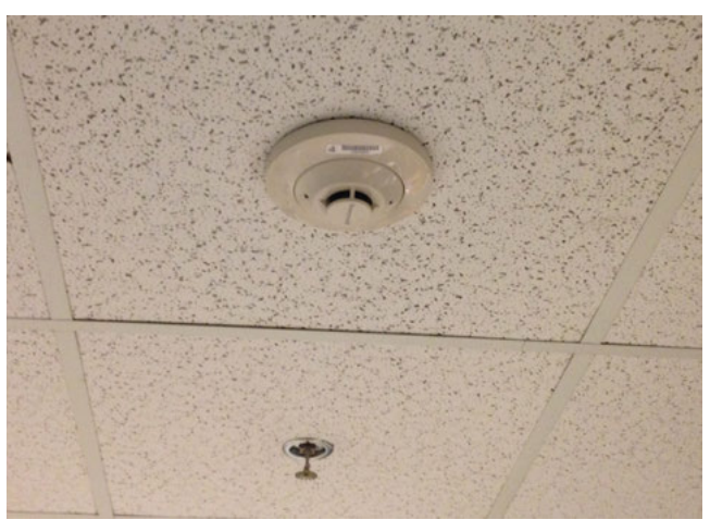
Smoke detector and sprinkler for alarm system initiation.
