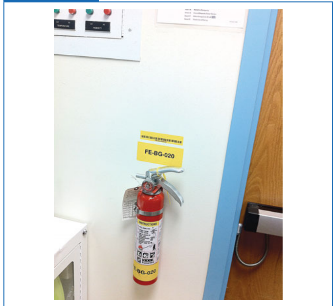
Portable fire extinguisher located in medical equipment servicing area.
