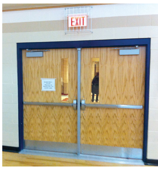
Exit sign with protective cover.
