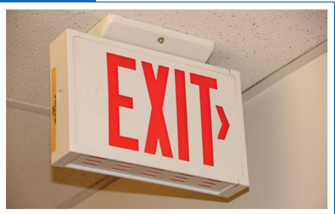
Directional exit sign.
