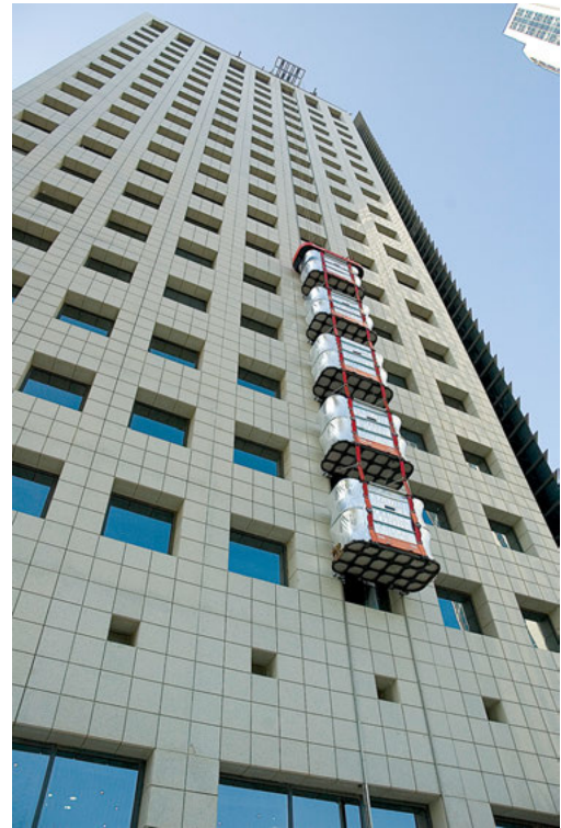
Roof-supported platform rescue system with multiple platforms installed on high-rise building. (Photo courtesy of Escape Rescue Systems, Ltd.)
