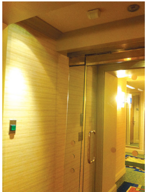
Egress side of access-controlled door assembly.
