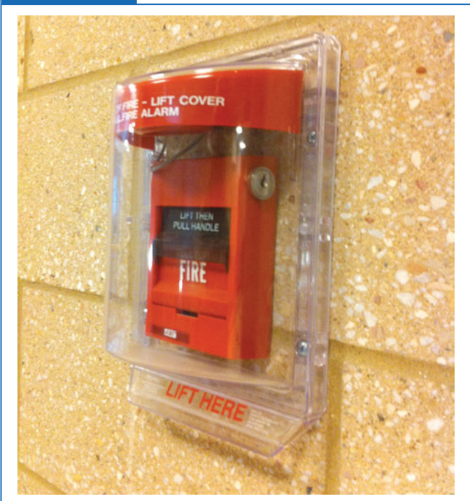
Manual fire alarm box with protective cover.
