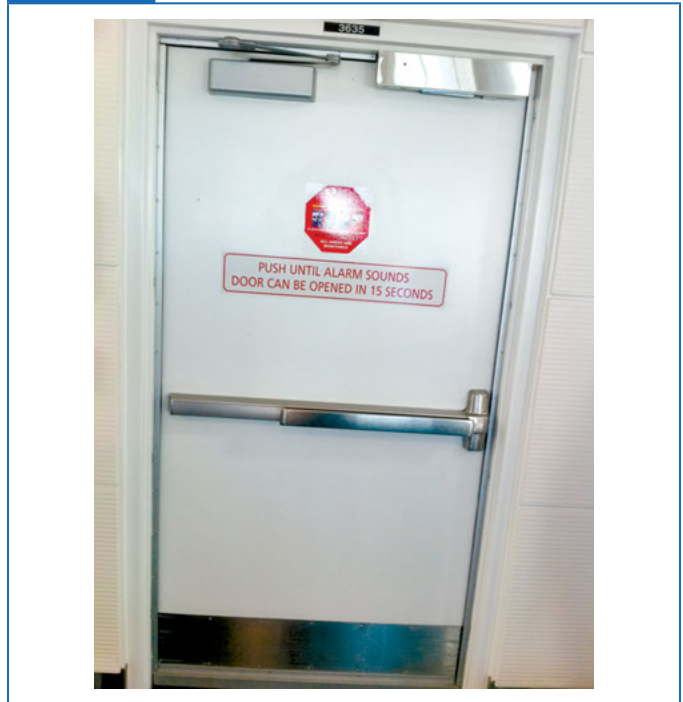
Delayed-egress locking hardware.
