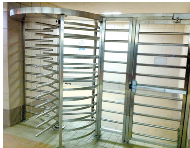
Assembly occupancy turnstile with required egress provided by gated, swinging door.
