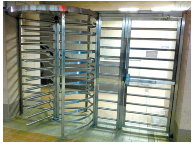
Panic hardware on non-rated, gated door opening.
