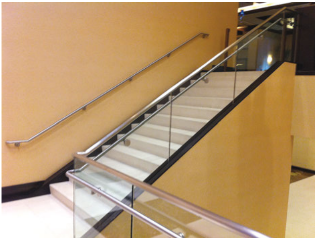
Unenclosed inside stair used as exit access.
