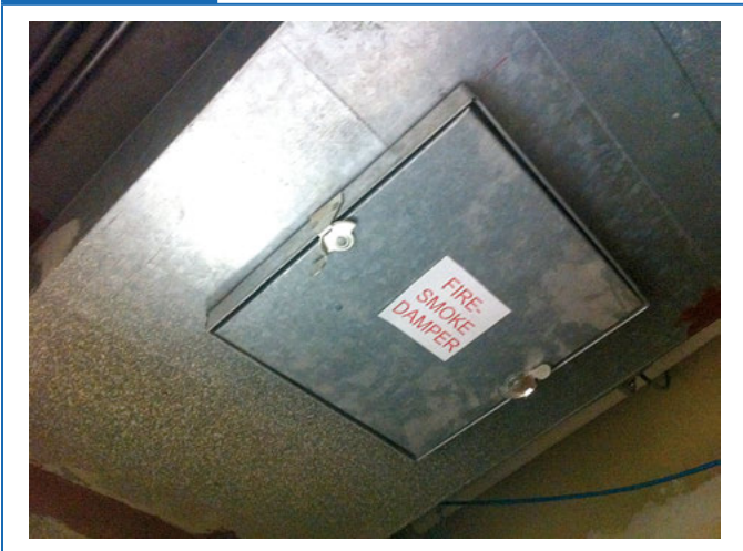
Smoke barrier duct penetration protected by smoke damper.
