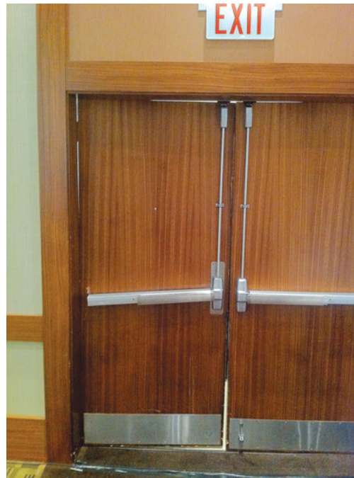
Damaged egress door subject to inspection.
