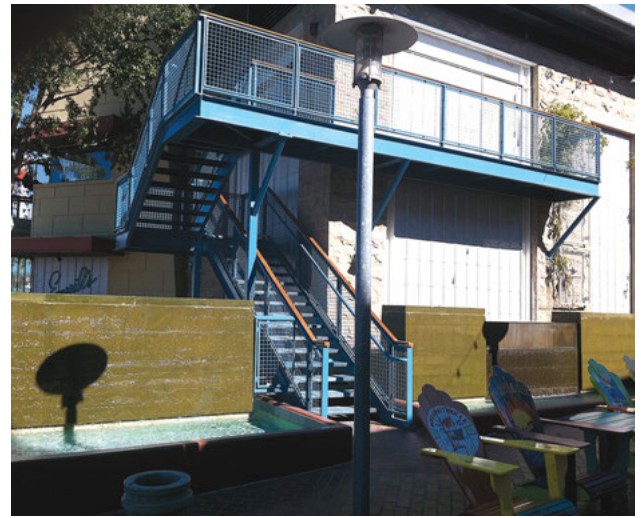
Guards at the open side of walking surfaces.
