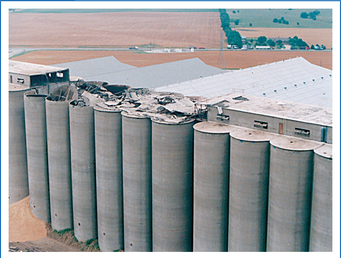
Explosion-damaged bulk storage facility.
