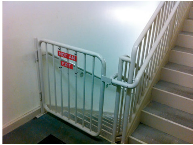
Egress stair, handrails, guards, and barrier to inadvertent travel past the level of exit discharge.
