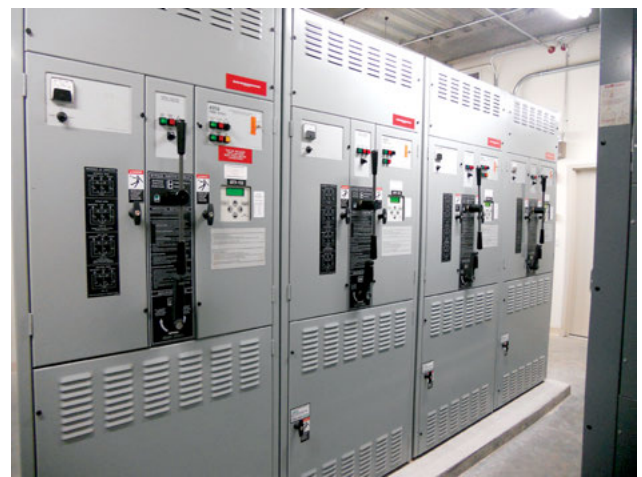
Emergency power distribution panels.
