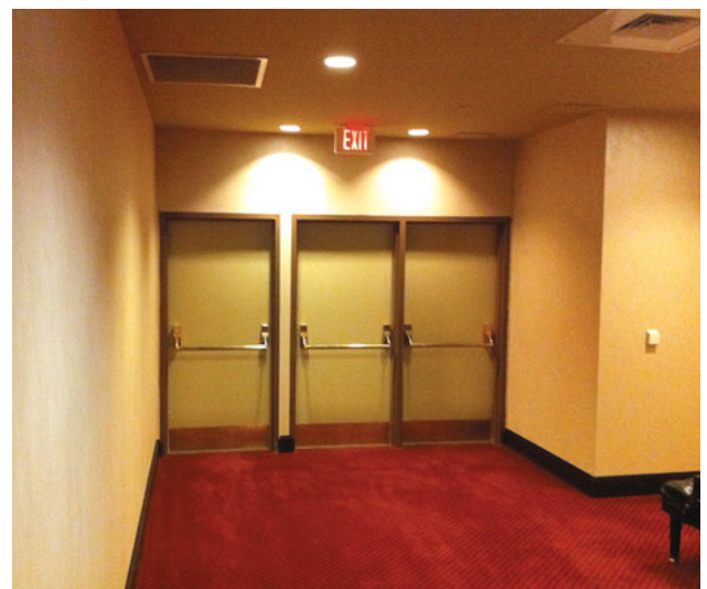
Fire exit hardware on fire door assemblies.
