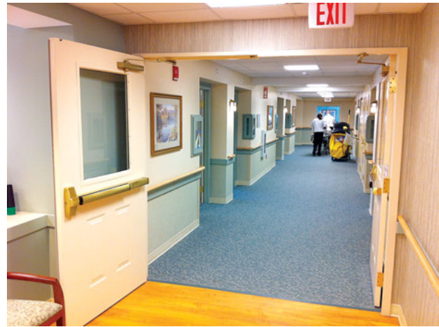
Smoke barrier door opening providing for patient relocation to safe smoke compartment.
