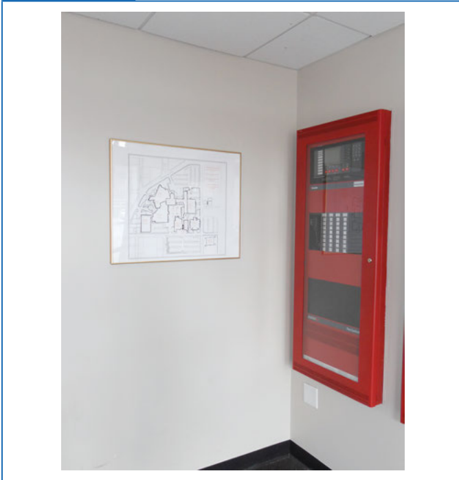
Alarm system annunciator panel on wall of minor entrance to hospital.
