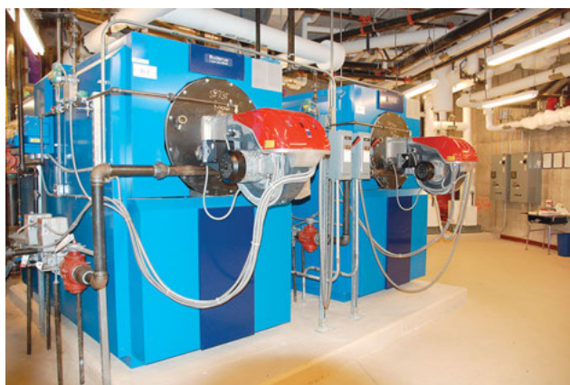
Boiler room requiring protection.
