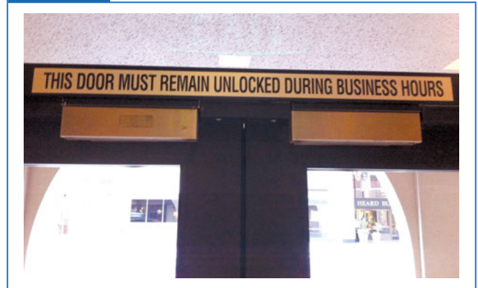
Sign over door subject to locking in an assembly occupancy.
