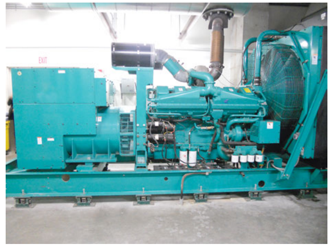
Hospital emergency power generator.
