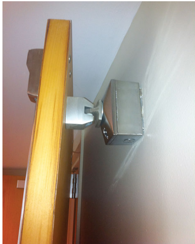
Hold-open mechanism on automatic-closing door.
