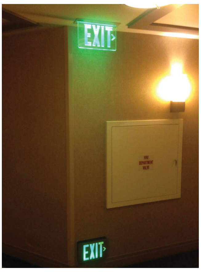
Two directional exit signs that are internally illuminated.
