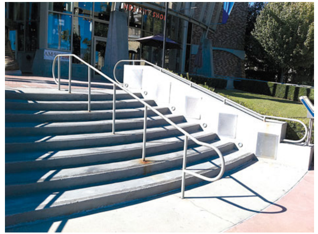
Outside stair used as exit discharge.
