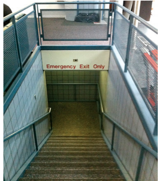
Guards at floor opening.
