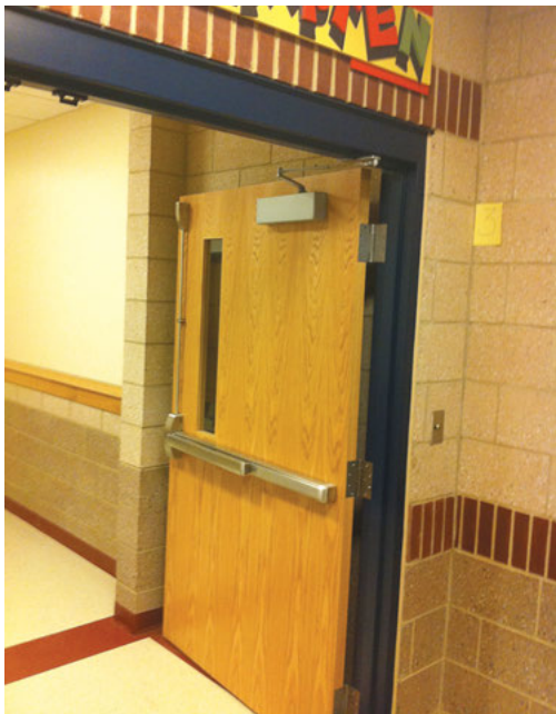
Fire-rated cross-corridor door with fire exit hardware.
