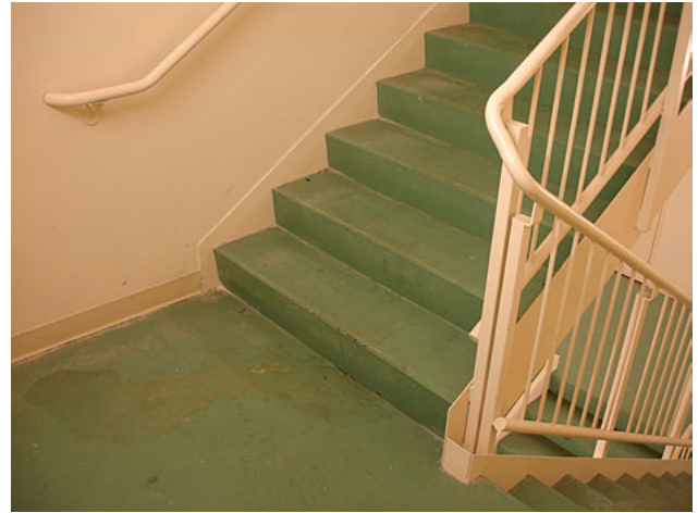
Continuous handrail on inside turn of stair at landing. (Photo courtesy of Jake Pauls)
