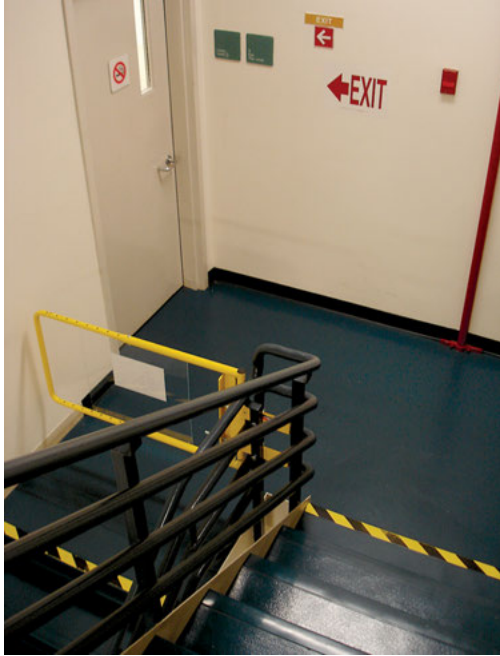
Interruption of exit stair at level of discharge. (Photo courtesy of Jake Pauls)
