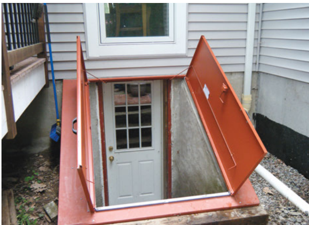
Bulkhead serving as secondary means of escape from a basement living area. (Photo courtesy of Bulkhead Doors, Inc.)
