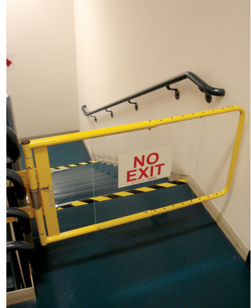
Sign on gate providing interruption of exit stair. (Photo courtesy of Jake Pauls)
