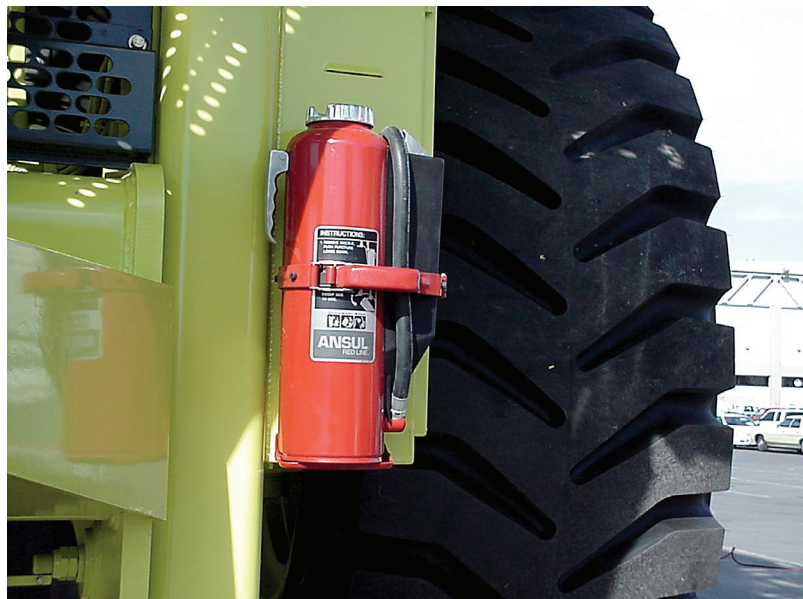
Exhibit 2(a) Extinguisher Installed on an Off-Road Vehicle. (Photo courtesy of Ansul Fire Protection, Inc.)
