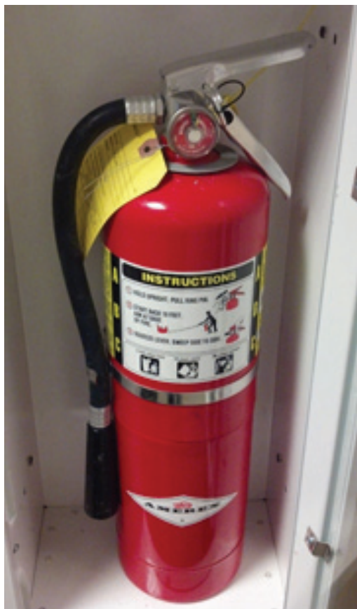
Exhibit 3 Inspection and Maintenance Tags on a Cabinet-Mounted Extinguisher.
