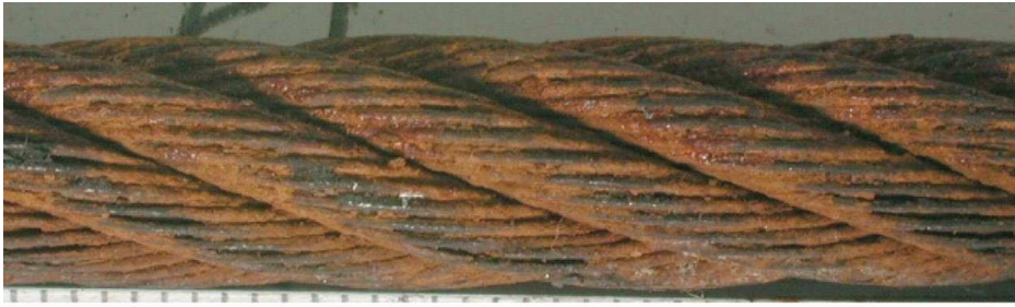
Figure I.4 — Surface heavily pitted and wires quite slack, gaps between wires — Discard immediately
