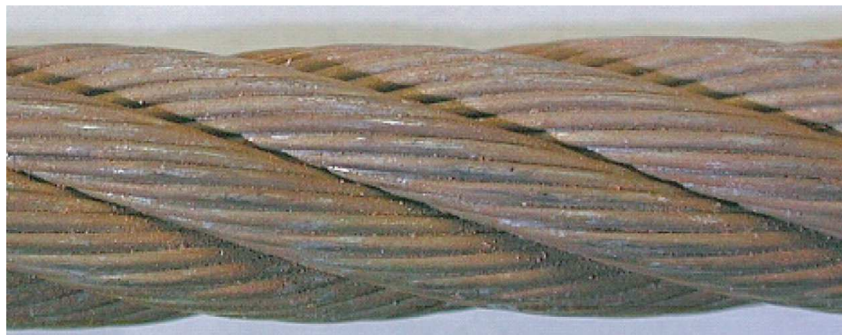
Figure I.1 — Beginning of surface oxidation, can be wiped clean, superficial — Rating: 0 % towards discard
