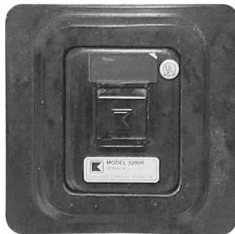
FIGURE 6.5.8.1 Typical Access Box.
